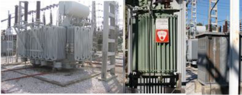
Fig. 2. Protected substation components: HV/MV Power Transformer (left), Neutral Reactance (centre) and Neutral Resistor (right)
