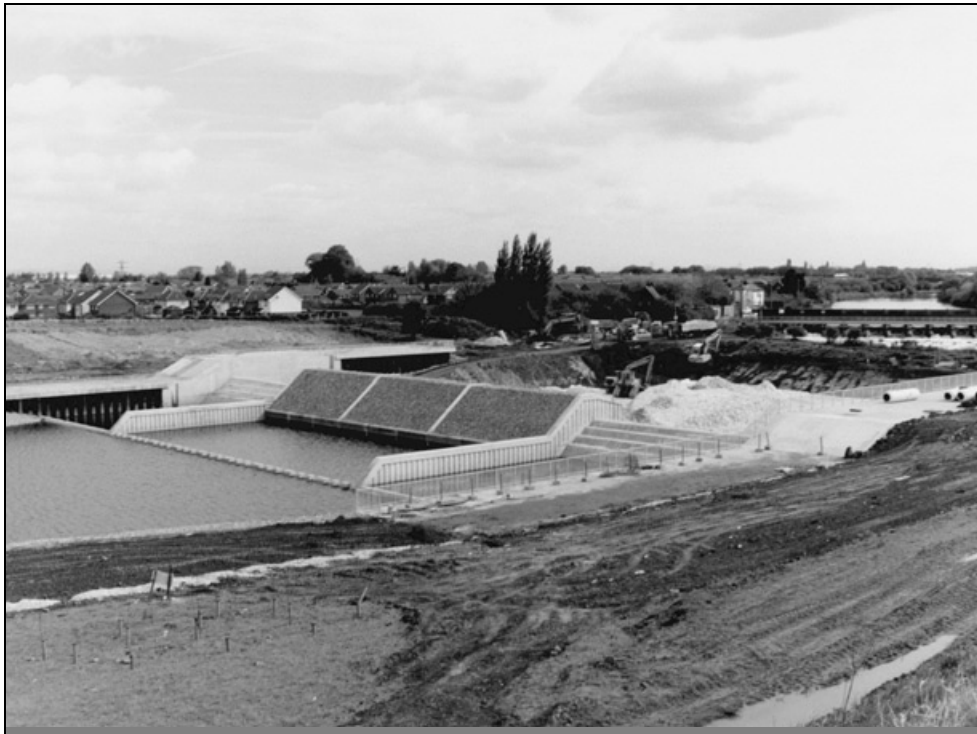
Fig. 11. View of weir from the south, near complete. Upstream erosion protection in progress
